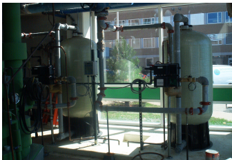
Newly Installed Regeneration Tanks at the Middleton VA Hospital
